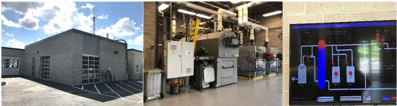
University of New Hampshire Thompson School of Applied Science Wood Chip District Heating System (Project details on page 24)
